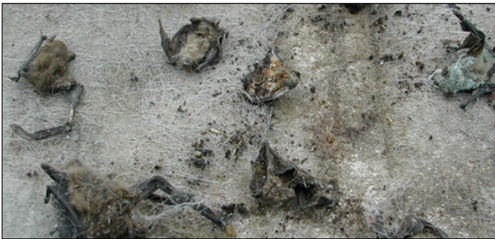
Dead bats trapped in breathable roof membrane
